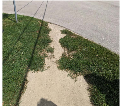
Deteriorating sidewalk with no curb ramp on Lannon Rd
