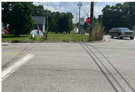
Missing sidewalk, crossing, and curb ramp at Good Hope Rd
