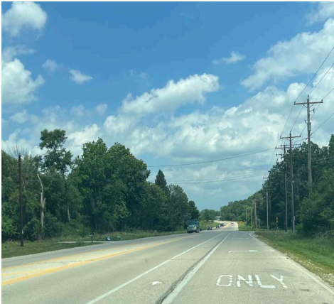
Faded bicycle lane markings on Main St
