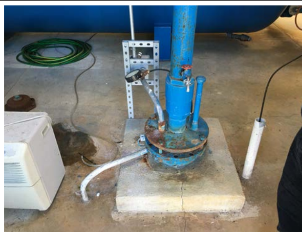
Figure 2.02-2 Well Discharge Piping
