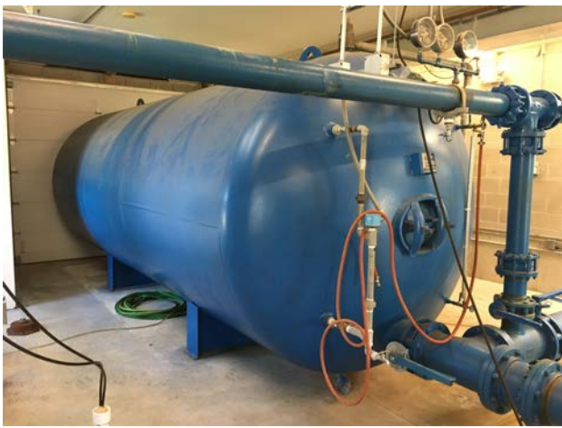
Figure 2.04-1 Pneumatic Pressure Tank
